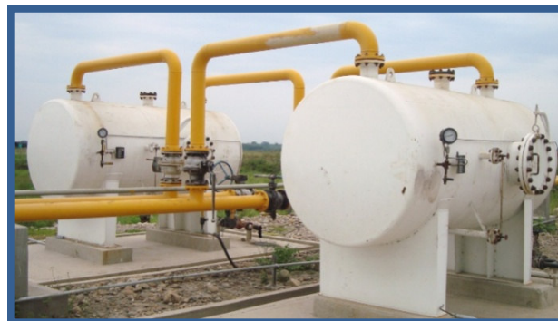
Foto 8.2. Knock Out Drum
