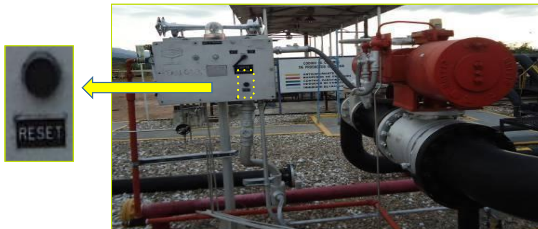
Figura 4. Tablero UL de la válvula Shut Down.
