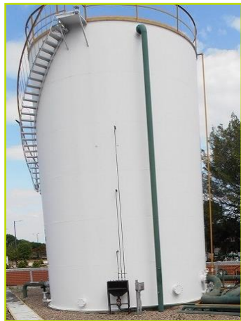
Figura No.43 Skimming Tank 3000-2
