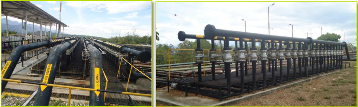
Figura No. 3 Manifold
