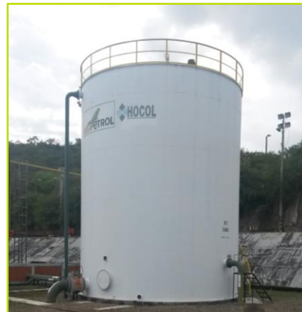
Figura No.44 Skimming Tank 5000-2
