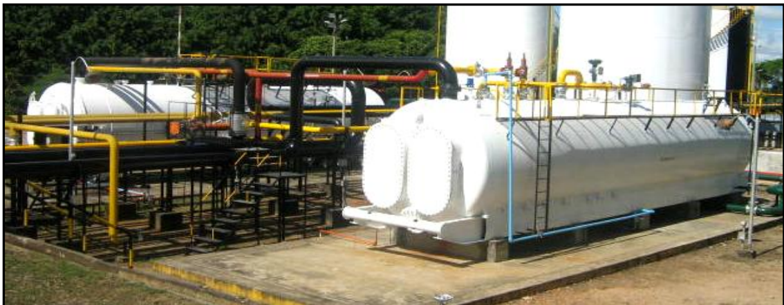
Figura 11. Free Water Knockout (FWKOs) (M-MAM-106/107)
